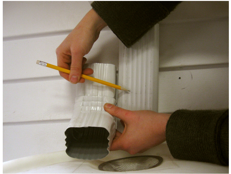
Figure 3. Marking the line where the downspout pipe will be cut and reconnected to the downspout elbow.
